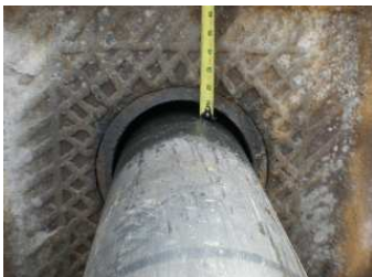
Worn Pin Bore
